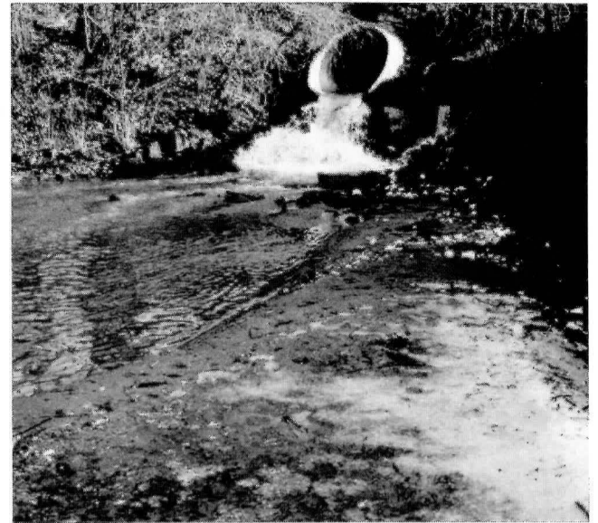
The Binnekill today: the route west has been filled in and these pipes discharge water from sources unknown to the author.
